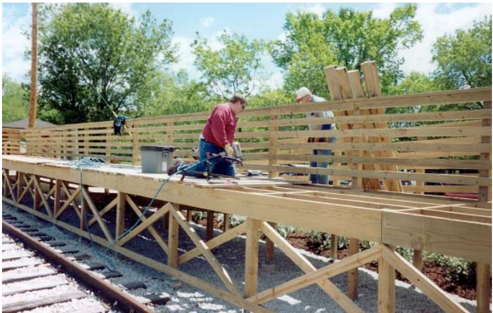
Mark Petersen and Ken Ward putting the finishing touches on the Blackhawk platform.
