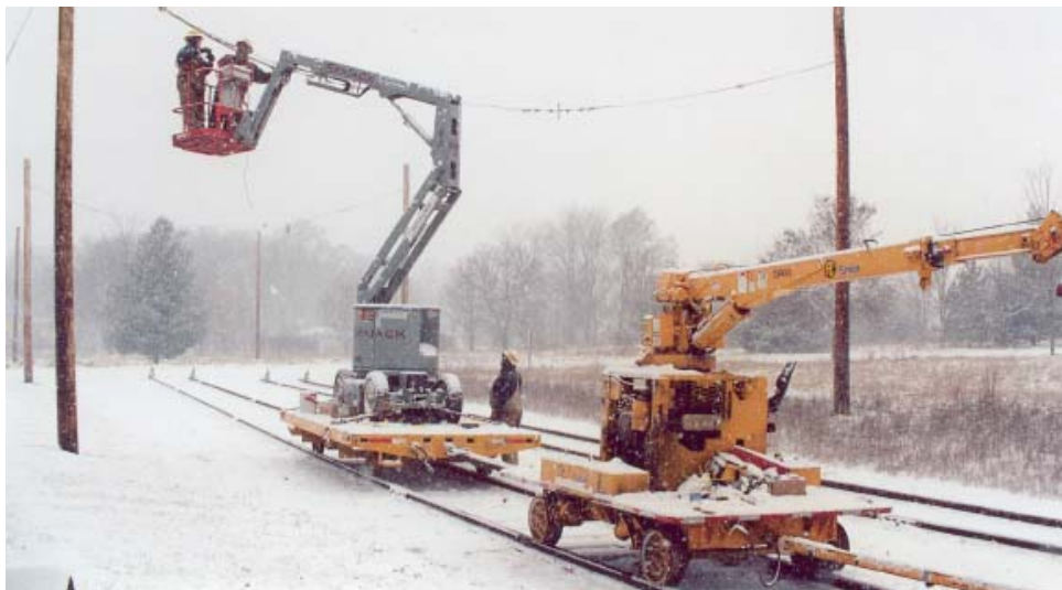
Placing of "span wires" from which the "trolley wire" is attached at Blackhawk.
