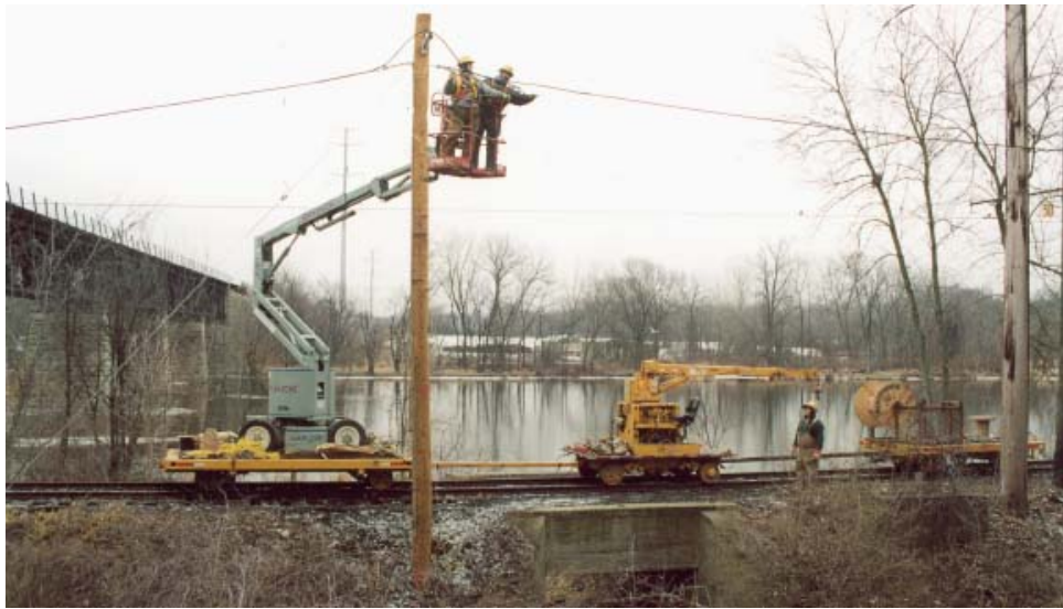
Supplying power to operate the museum's cars on the extension required the installation of a "600 v. feeder line" from Castlemuir on the north to the extension as well as "trolley wire" over the tracks. Seen here are the men and equipment installing the "feeder line" just south of the Canadian National bridge.
