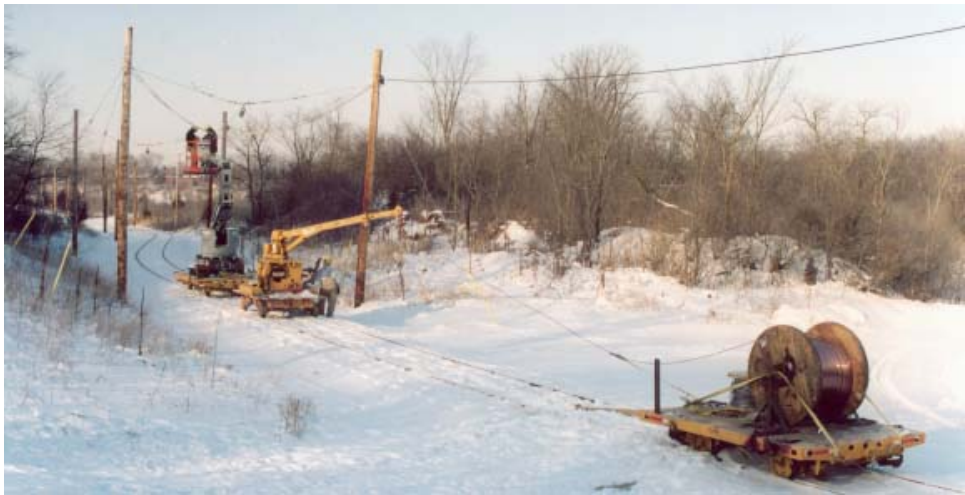
Stringing "trolley wire" near the pond. Note the "feeder line" and the reel of shiny "trolley wire."
