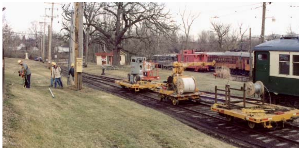
The Aldridge Contractor's equipment and their crew at Castlemuir working on the "feeder line."
