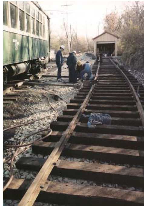
Looking towards the "MOW" on Track One West prior to ballasting - October 2001.
