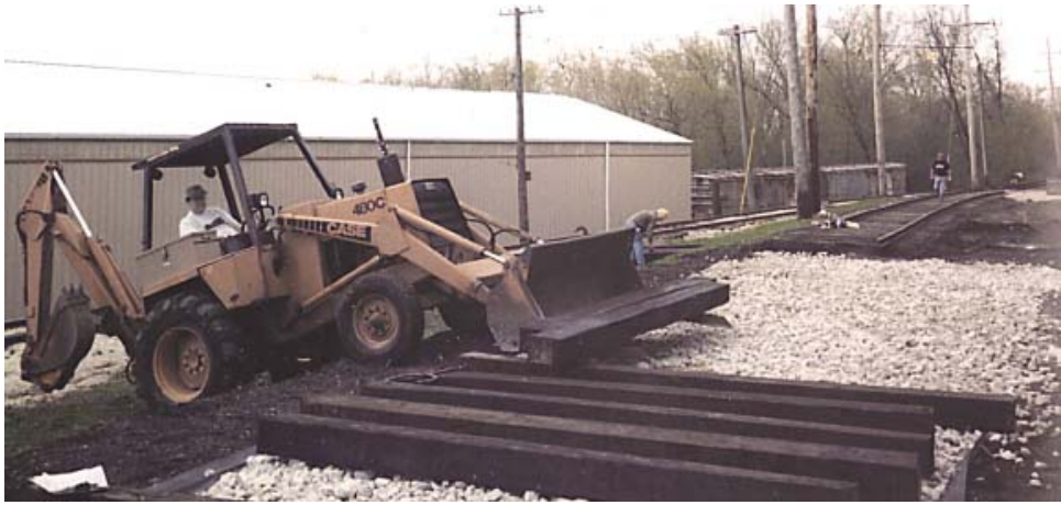
The mainline is cut and switch ties being placed for track one west. Fred Lonnes at the controls of the front end loader - April 2001.
