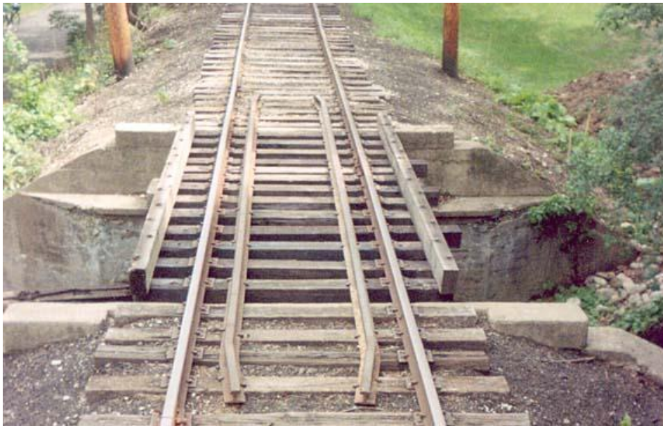
Ward's Bridge with new "guard rails" installed this summer. Picture is looking south.
